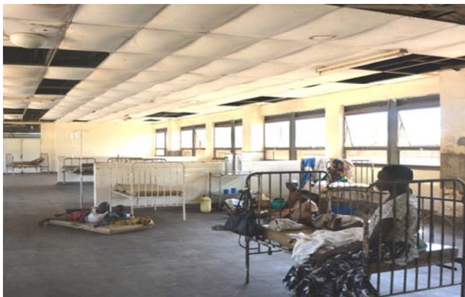
Children in the dilapidated Abim Referral Hospital Paediatric Ward
